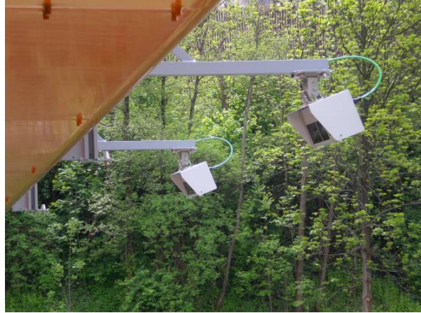
Figure 10: Fixing of the CALM-IR transceivers on a VMS gantry at the Austrian COOPERS test site
